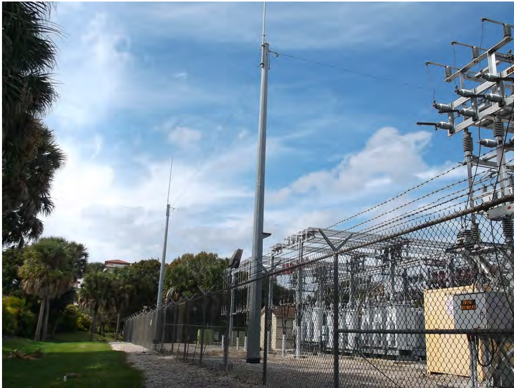
Photo #2: View of the existing lightning shielding mast which will be replaced facing west.
