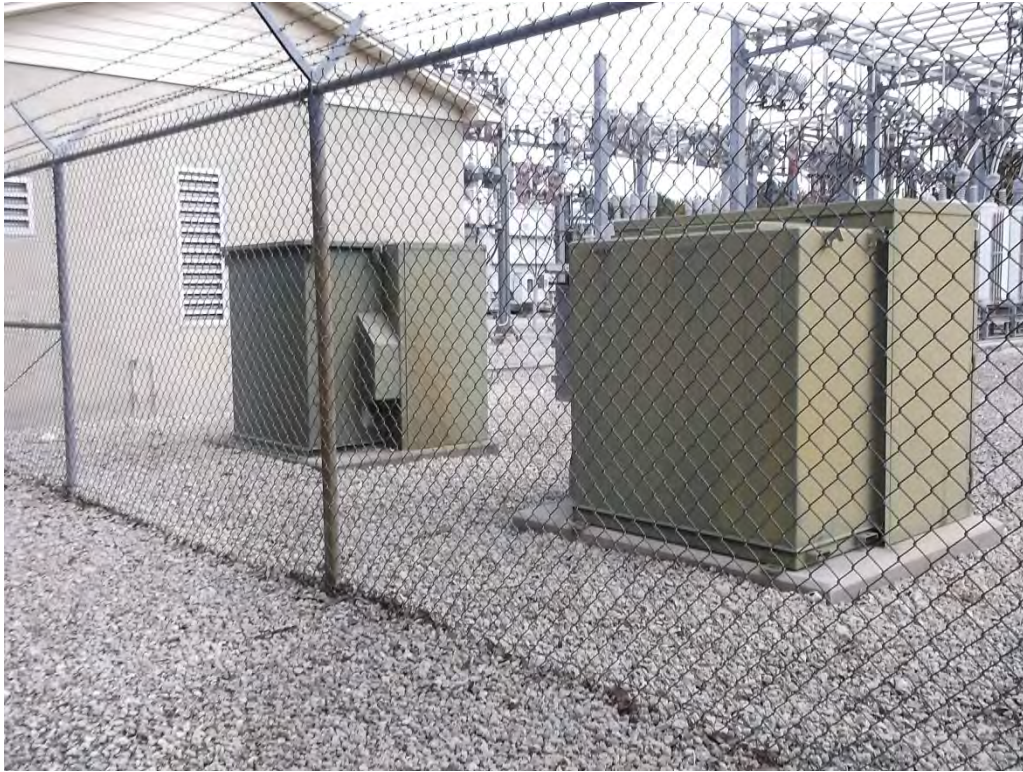
Photo #5: View of the pad-mounted transformers observed in the southwestern portion of the substation.
