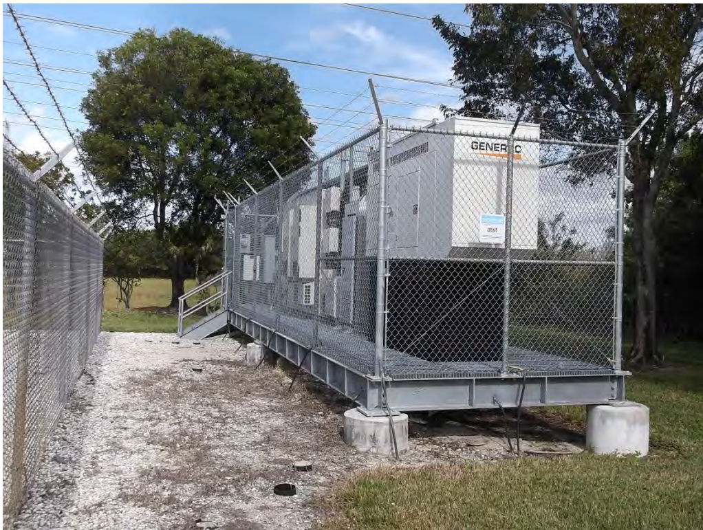
Photo #8: View of the AT&T equipment lease area at the northeast corner of the substation facing north.
