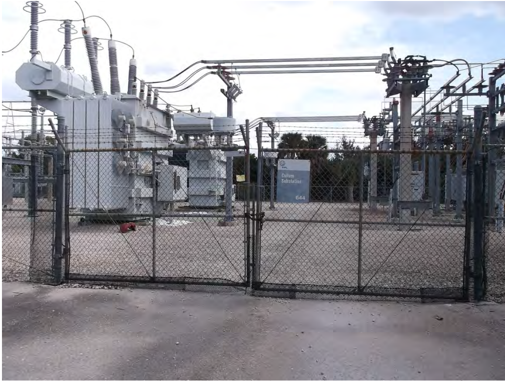
Photo #1: View of the parent parcel and substation facing east.
