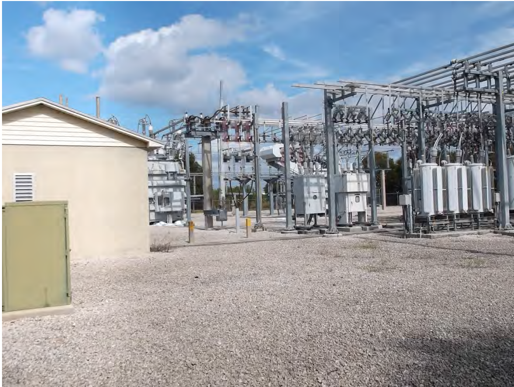
Photo #7: View of the parent parcel and substation facing northeast.
