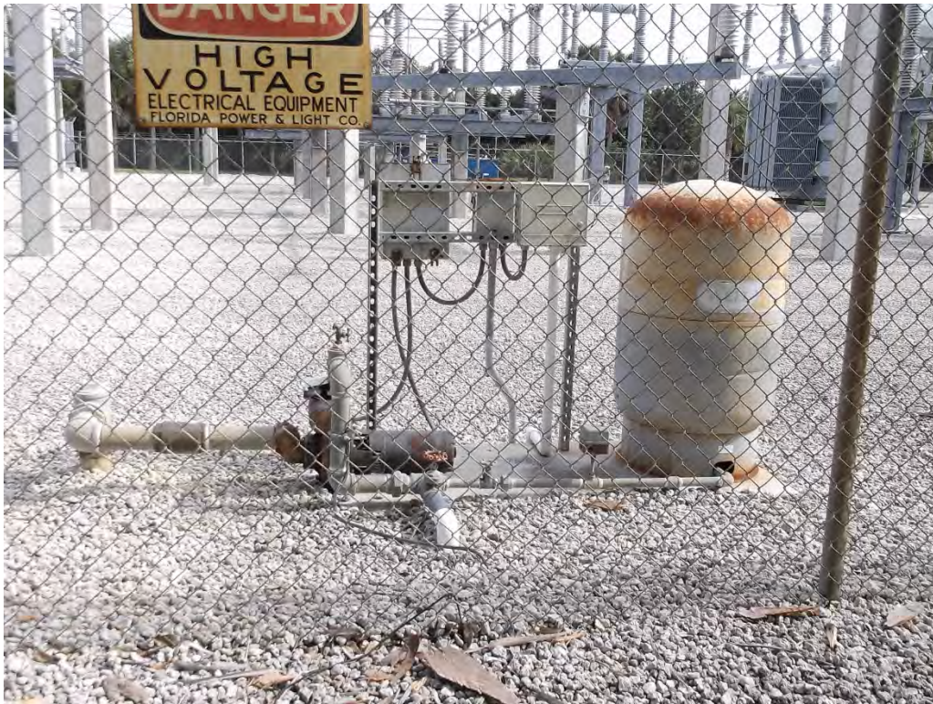
Photo #6: View of the well observed in the western portion of the substation.
